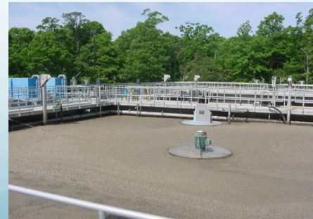
Sewage Treatment Plants
